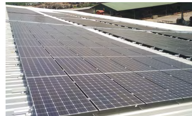
Malaysia Trapezoid Metal Roof 500KW
