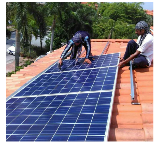
Malaysia Tile Roof 500KW
