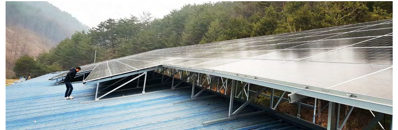
250KW Roof South Korea
