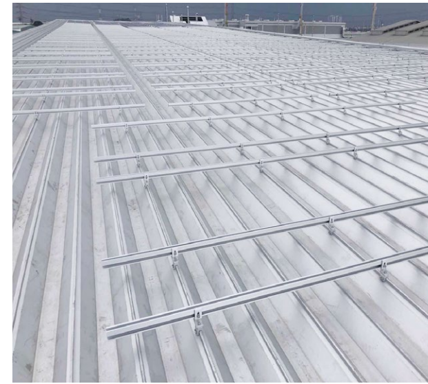
2MW Malaysia Kawa Roof
