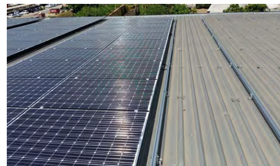
200KW Metal Roof Malaysia
